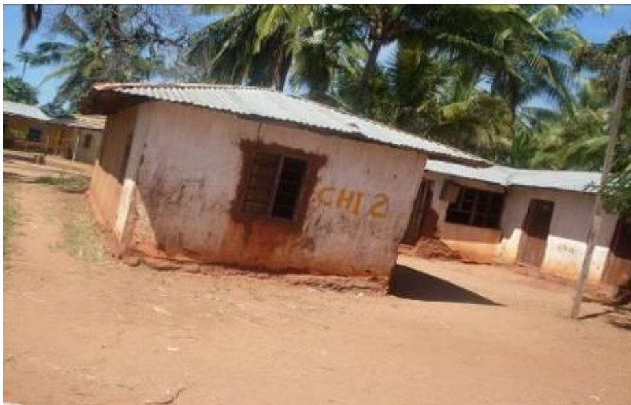
Figure 11-2: Chipuputa Village Council Office- One of the affected public buildings
