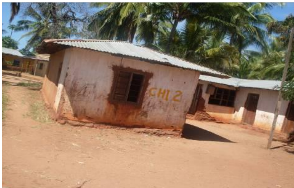
Figure 8-8: Chipuputa Village Council Office- One of the affected public buildings
