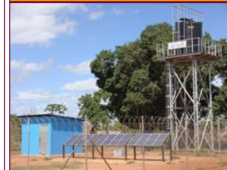
Systems powered by solar energy
