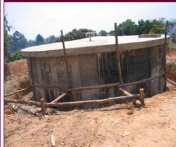
Ground Water Tank for Gravity Flow Scheme in Mzimba, Malawi
