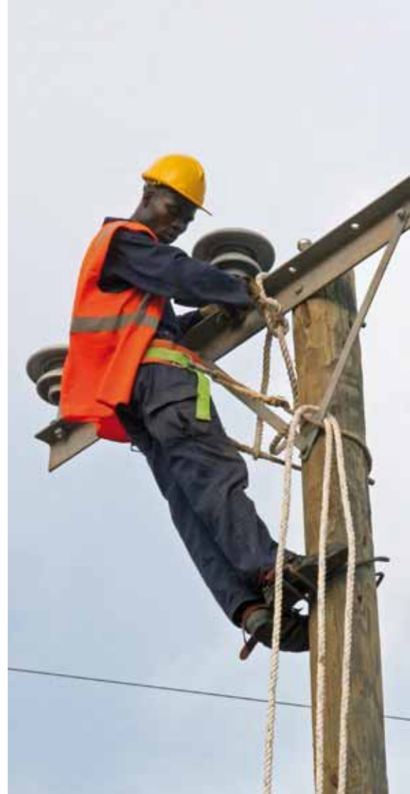
A man works on an electricity pylon in Liberia Photo © Betty Press / Panos
