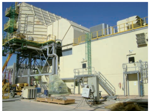
Ain Beni Mathar Solar Thermal Power Station
