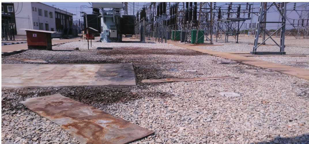
Plate 4.3.6 showing the location of the faulted Orange Grove transformer
