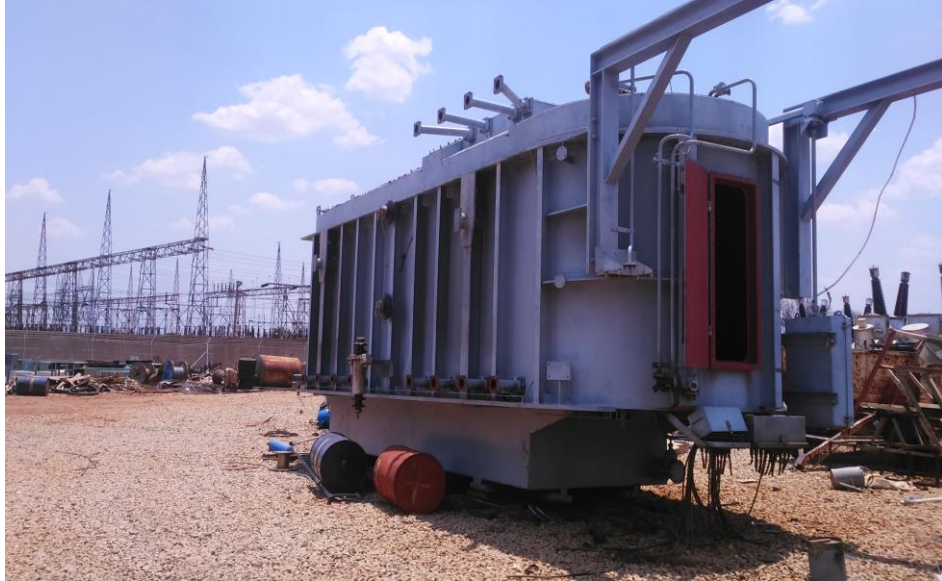
Plate 4.3.5 showing the faulted Sherwood transformer which was de-tanked
