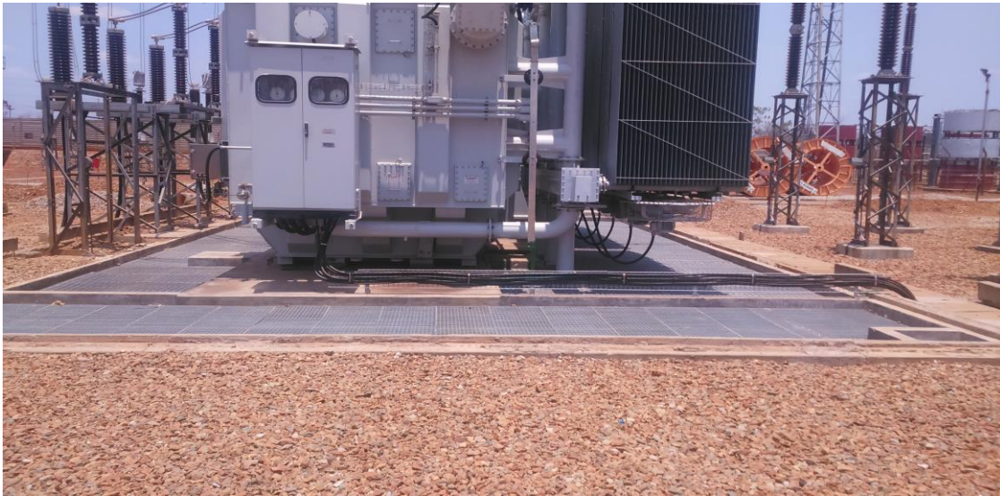
Plate 4.3.7 showing bunding around one transformer at Sherwood
