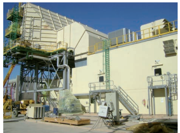
Ain Béni Mathar, installation thermo-solaire
