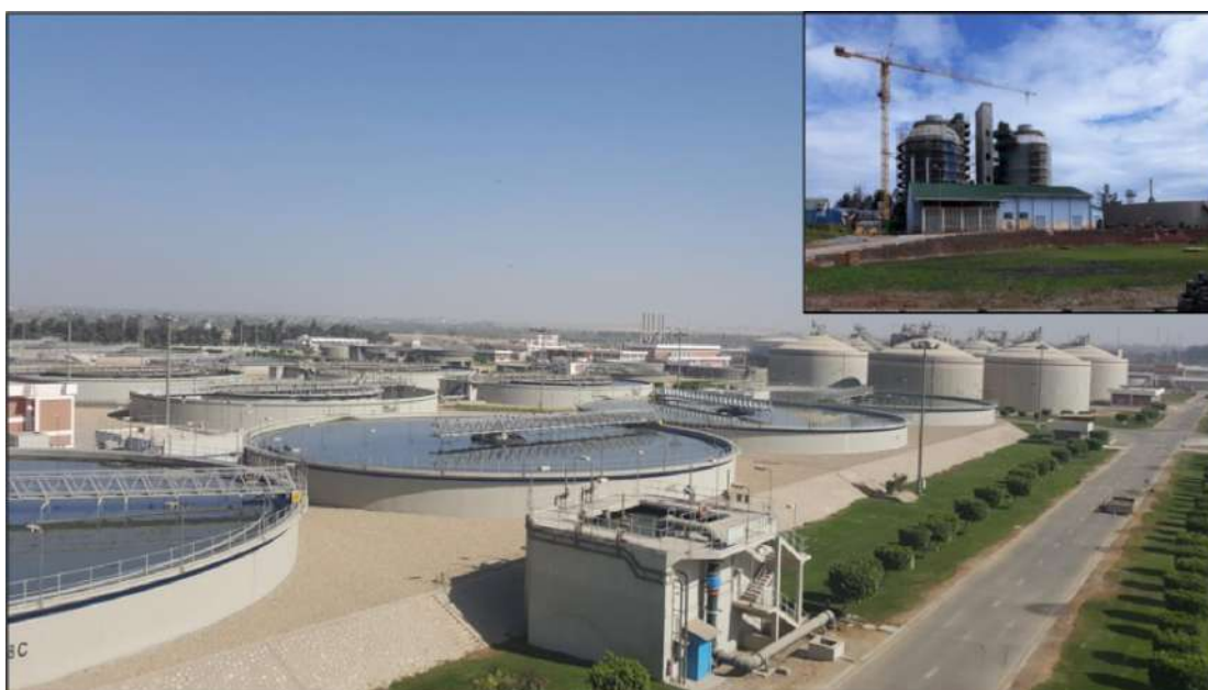
EGYPT- Gabal El-Asfar Wastewater Treatment Plant. In the background are anaerobic sludge digesters for energy production. Inset are similar digesters at a smaller wastewater treatment plant in Kampala. Anaerobic sludge digestion with energy recovery is a cost-effective and environmentally friendly option for sludge stabilization. The treated sludge can be used to increase soil productivity and crop yields.
