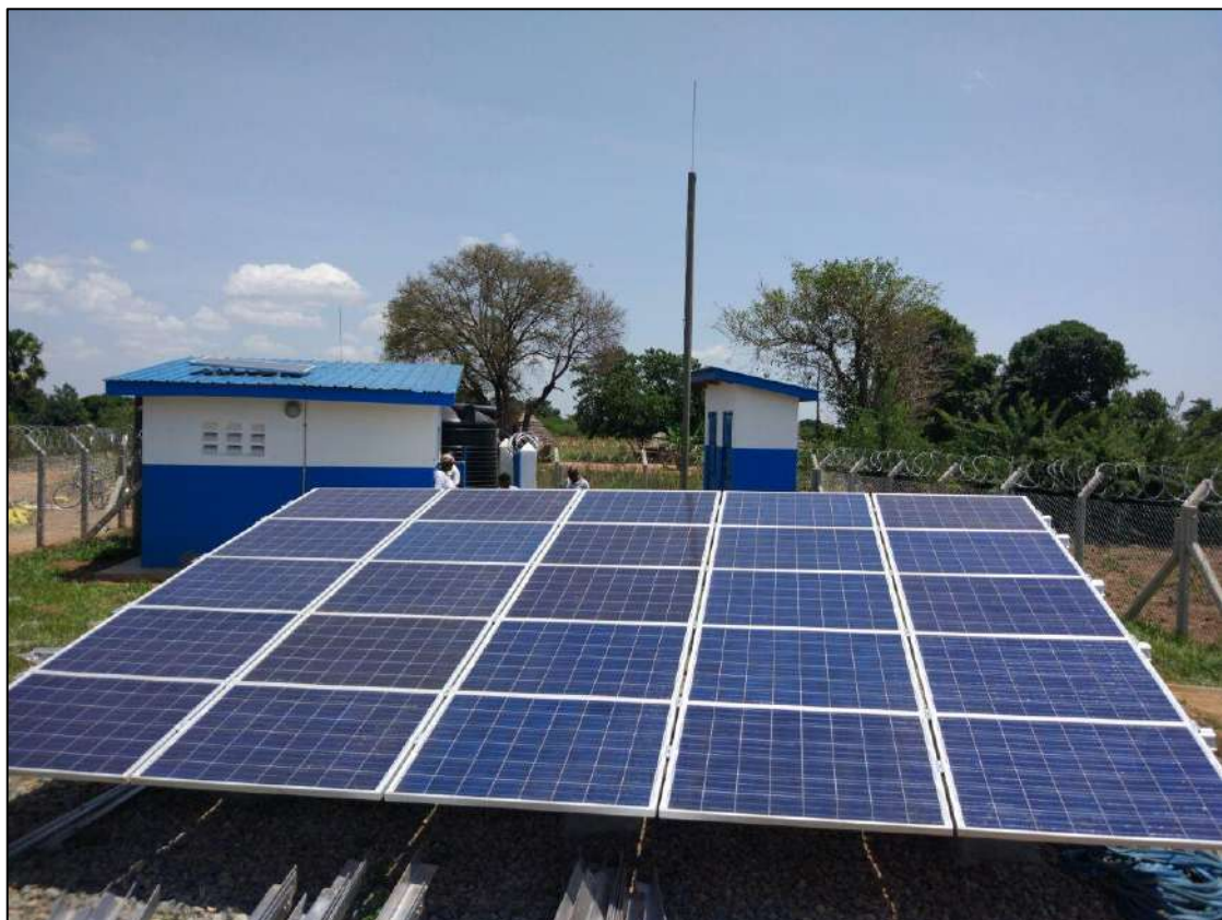
UGANDA -Ngora Solar Water Pumping System. Bringing water closer to people’s homes calls also for greater investments in energy and infrastructure. Solar and wind energy are increasingly used for water supply in Africa e.g. in Egypt, Ethiopia, The Gambia, Kenya, Morocco, South Africa and Tanzania.
